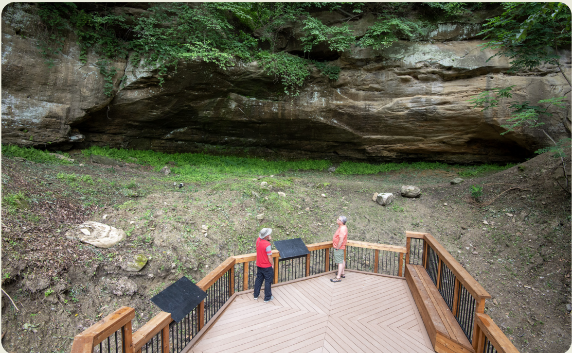
A new boardwalk and deck replaced a failing structure, giving visitors an up-close look at the iconic cave at Indian Cave State Park in Richardson County, while also protecting the historic petroglyph etchings. Visitors can reach the deck at the base of the cave via a stair tower or a ramp that is compliant with the Americans with Disabilities Act.
