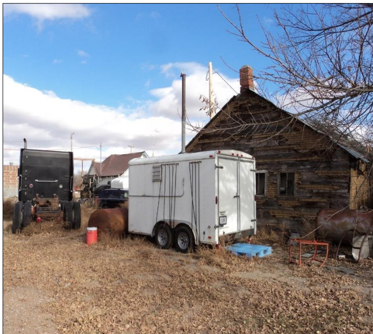
Air sparge/soil vapor extraction remediation system at the site of a former gas station.
