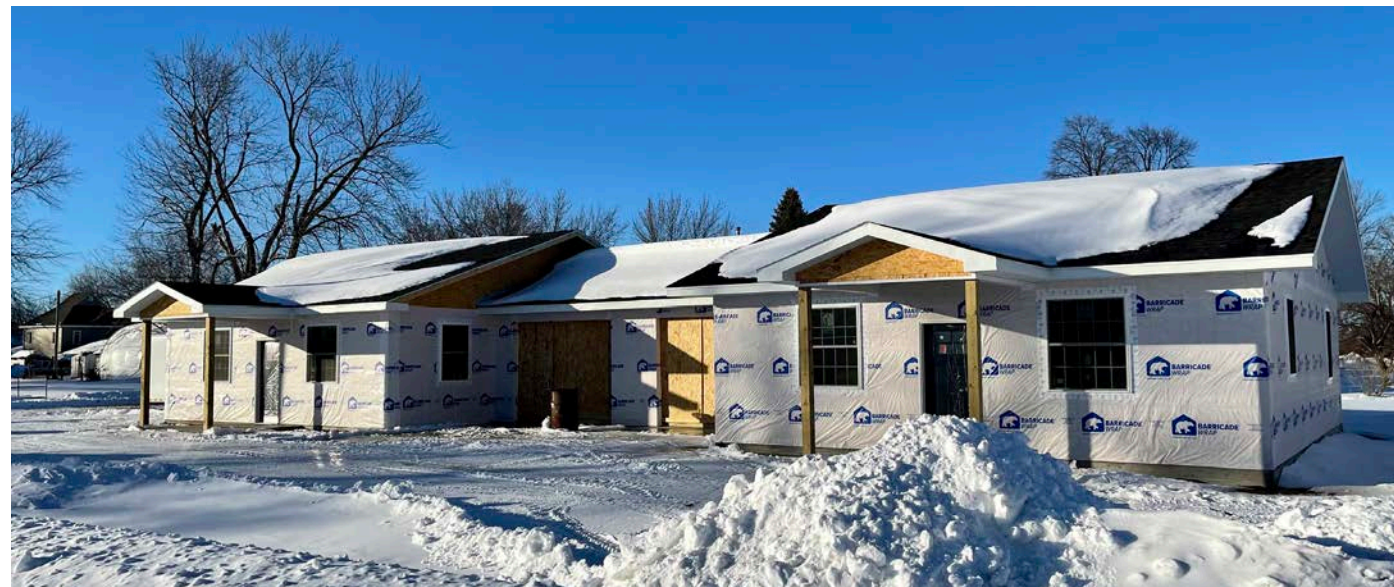
Construction moves forward on the NAHTF duplex project in the Village of Clearwater.
