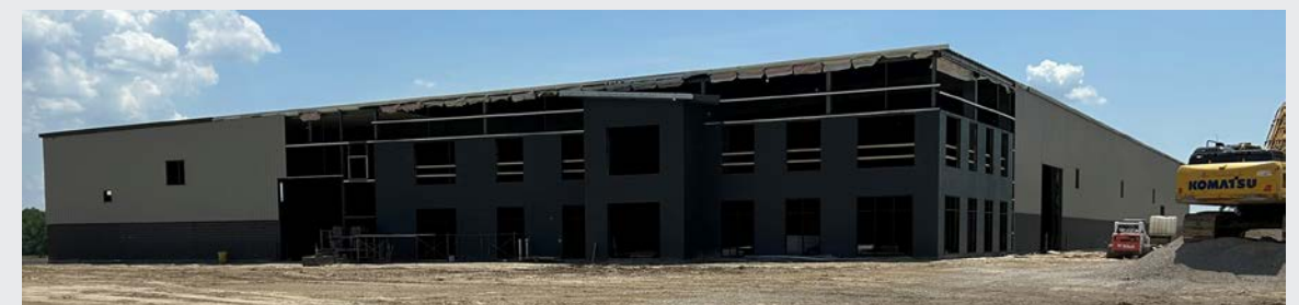
Construction in progress at the new Wearparts facility in Gothenburg Industrial Park
