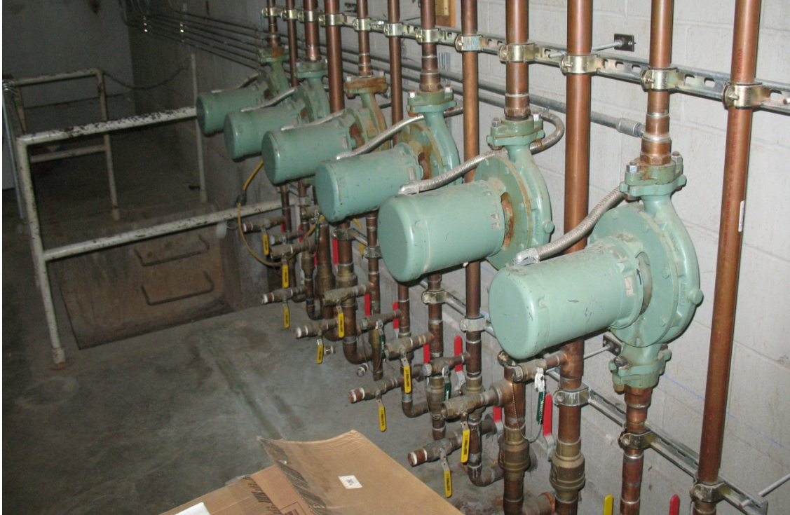
Geothermal Heating Pumps in Mechanical Area
