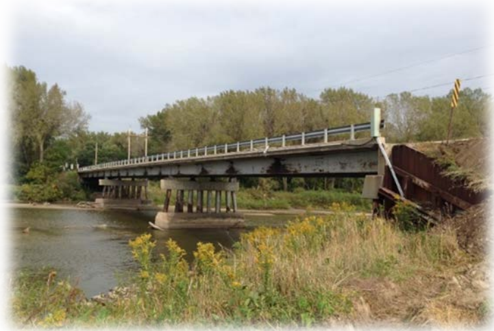
THE TRANSPORTATION AND TELECOMMUNICATIONS COMMITTEE VISITED THIS BRIDGE SOUTH OF BEEMER THAT WASHED OUT DURING THE 2010 ELKHORN RIVER FLOOD, WHICH CUT OFF ACCESS TO THE TOWN FOR SEVERAL MONTHS.
