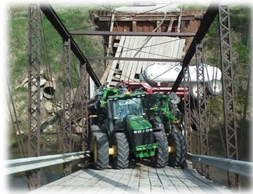
A SPRAYER IS TOO HEAVY FOR A RURAL BRIDGE IN OTOE COUNTY.
