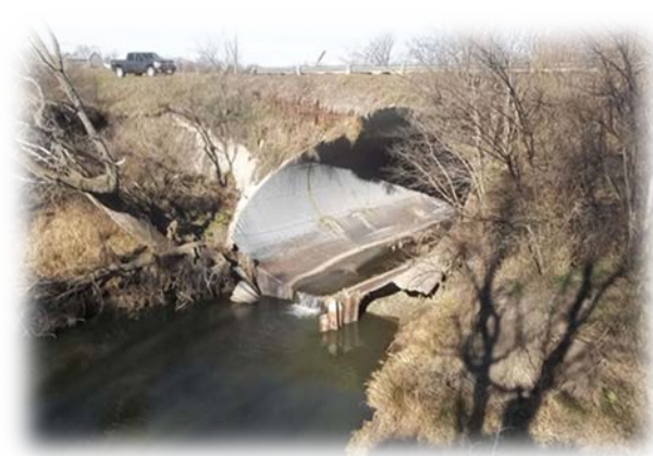
DEGREDDATION OF WOLF CREEK IS EVIDENT AS THE CHANNEL HAS DROPPED SIGNICANTLY BELOW A LARGE CULVERT UNDER COUNTY ROAD “I”, WEST OF SYRACUSE IN OTOE COUNTY.
