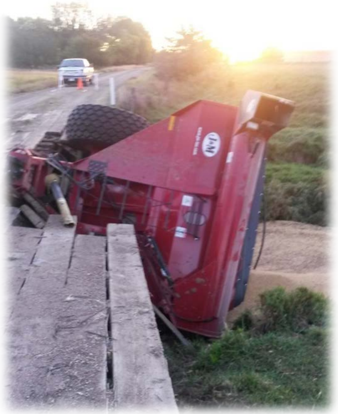
A NANCE COUNTY BRIDGE COLLAPSES UNDER THE WEIGHT OF AN AGRICULTURAL TRAILER IN 2014.
