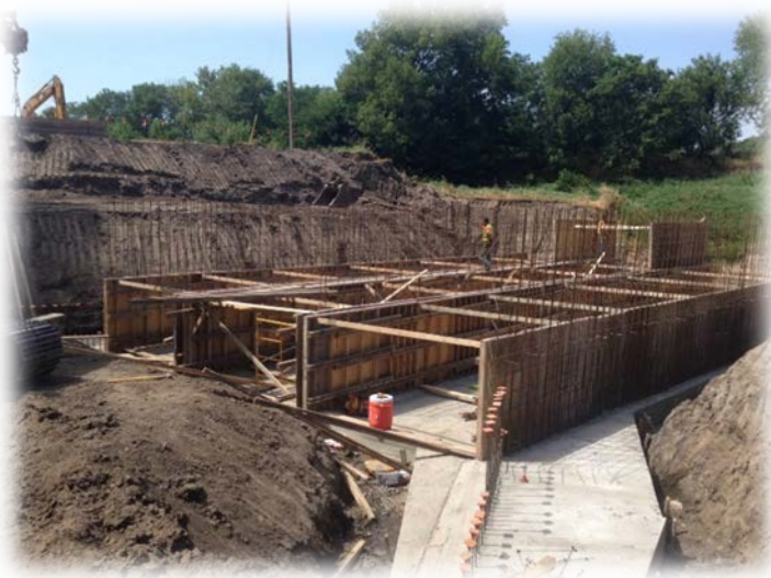
A RURAL BRIDGE IN OTOE COUNTY IS BEING REPLACED WITH THIS BOX CULVERT UNDER CONSTRUCTION.
