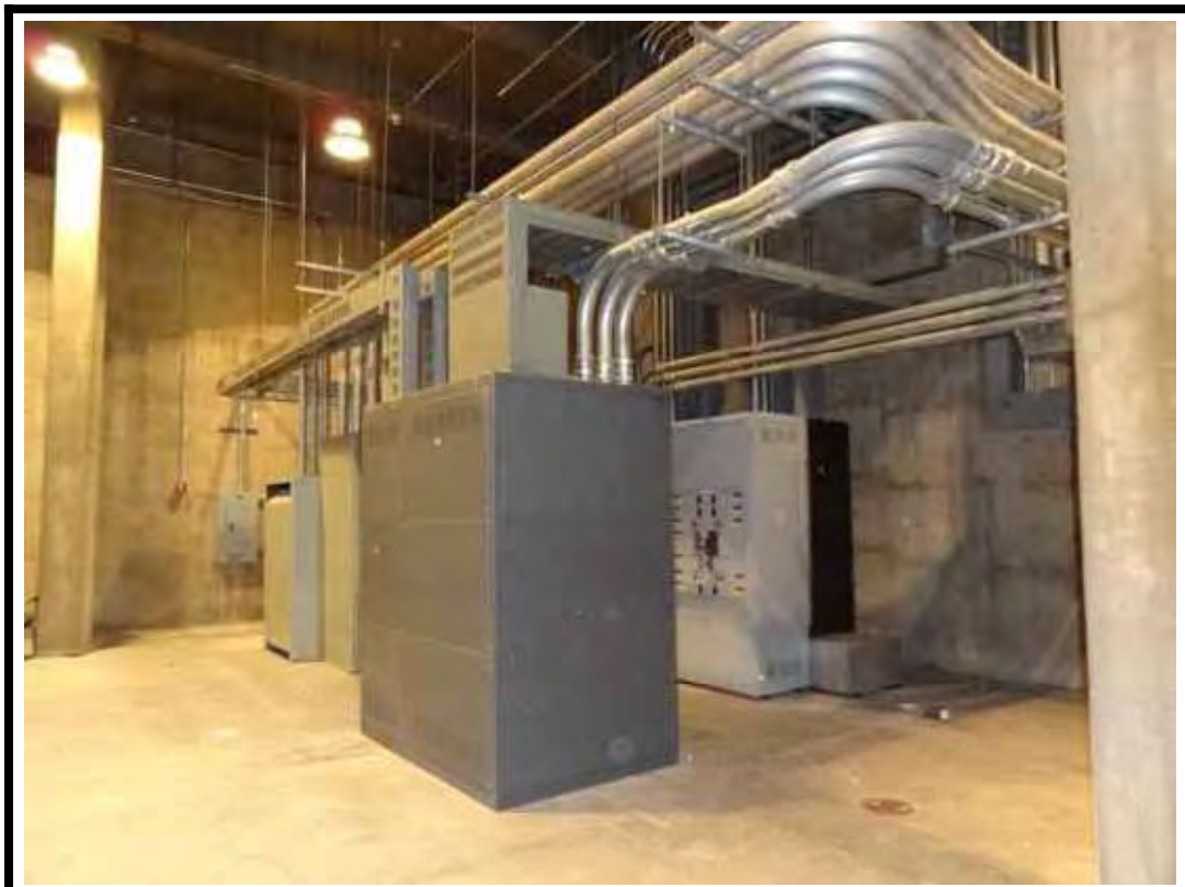
PHOTO NUMBER 46 View of electrical room in the subbasement.
