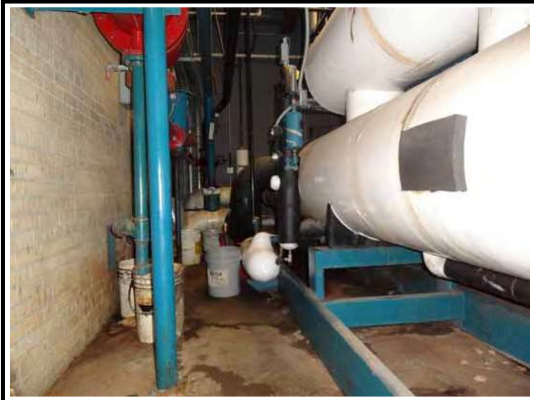
PHOTO NUMBER 81 View of the ice making equipment.
