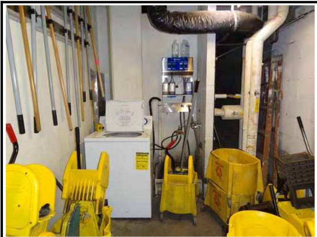
PHOTO NUMBER 8 View of one of several janitor's closets in the Civic Auditorium.
