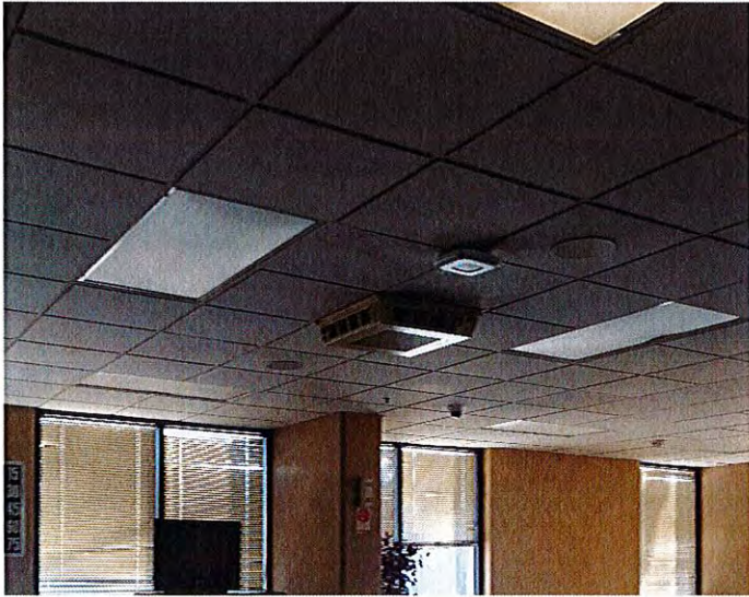
Lighting and ceiling
