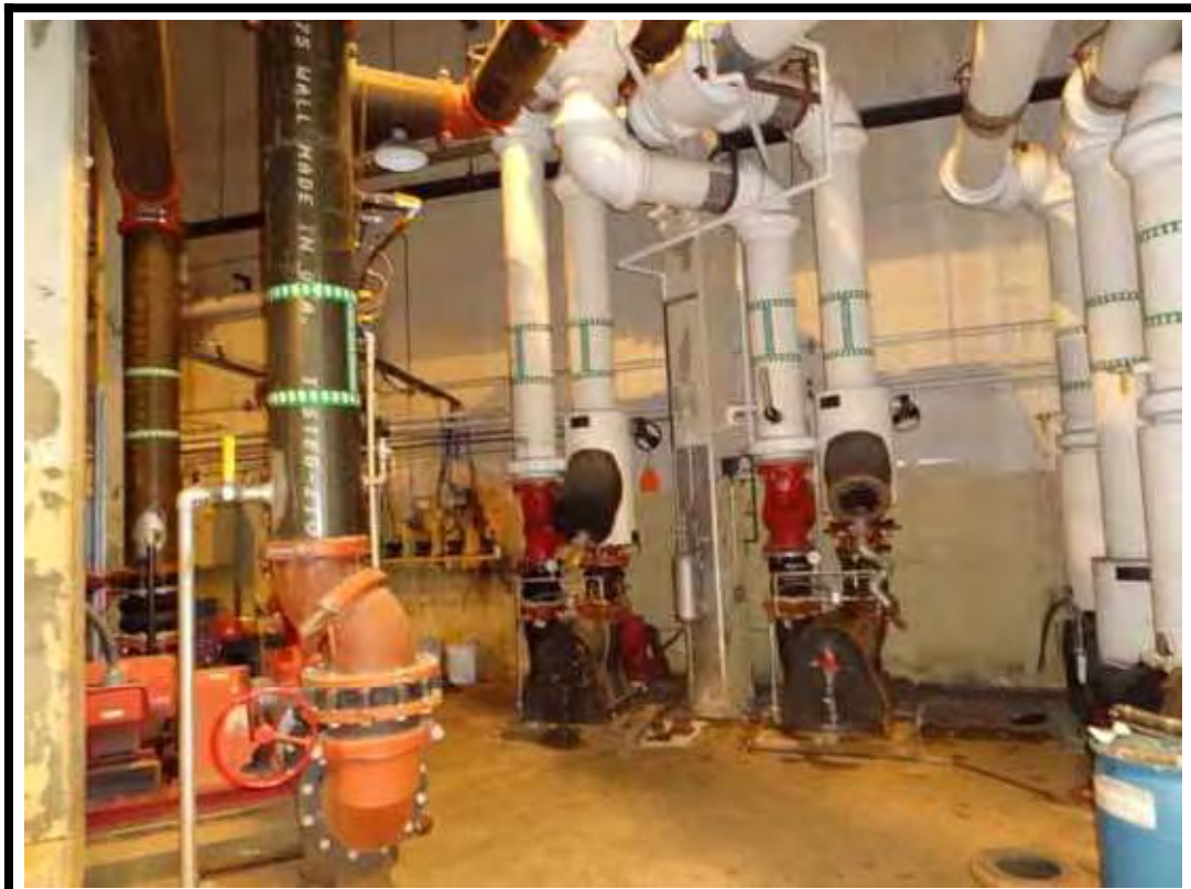
PHOTO NUMBER 66 View of water pipes in the subbasement.
