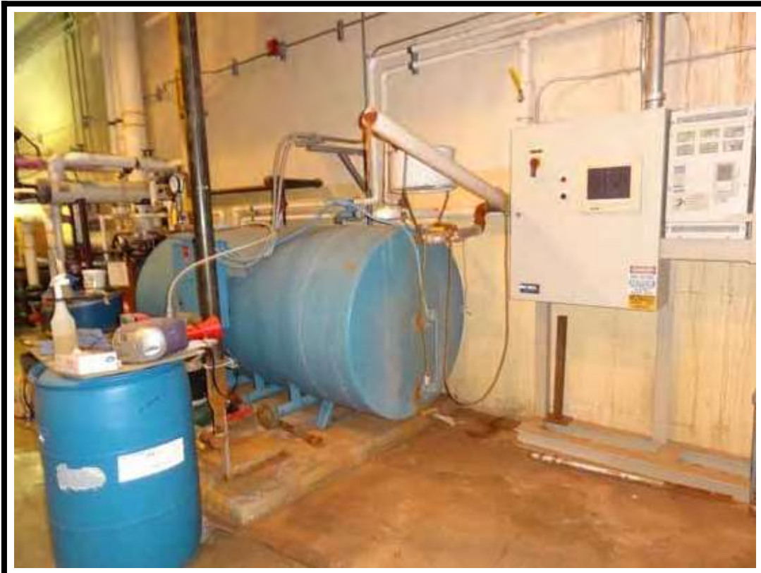
PHOTO NUMBER 59 View of water tank in the subbasement.
