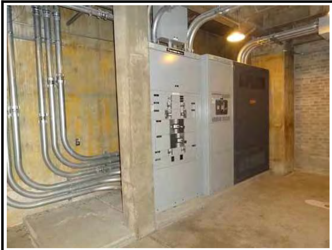
PHOTO NUMBER 73 View of electrical room in the basement.
