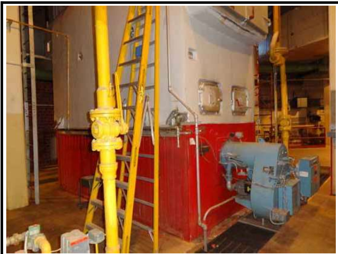
PHOTO NUMBER 60 View of one of two boilers in the subbasement.
