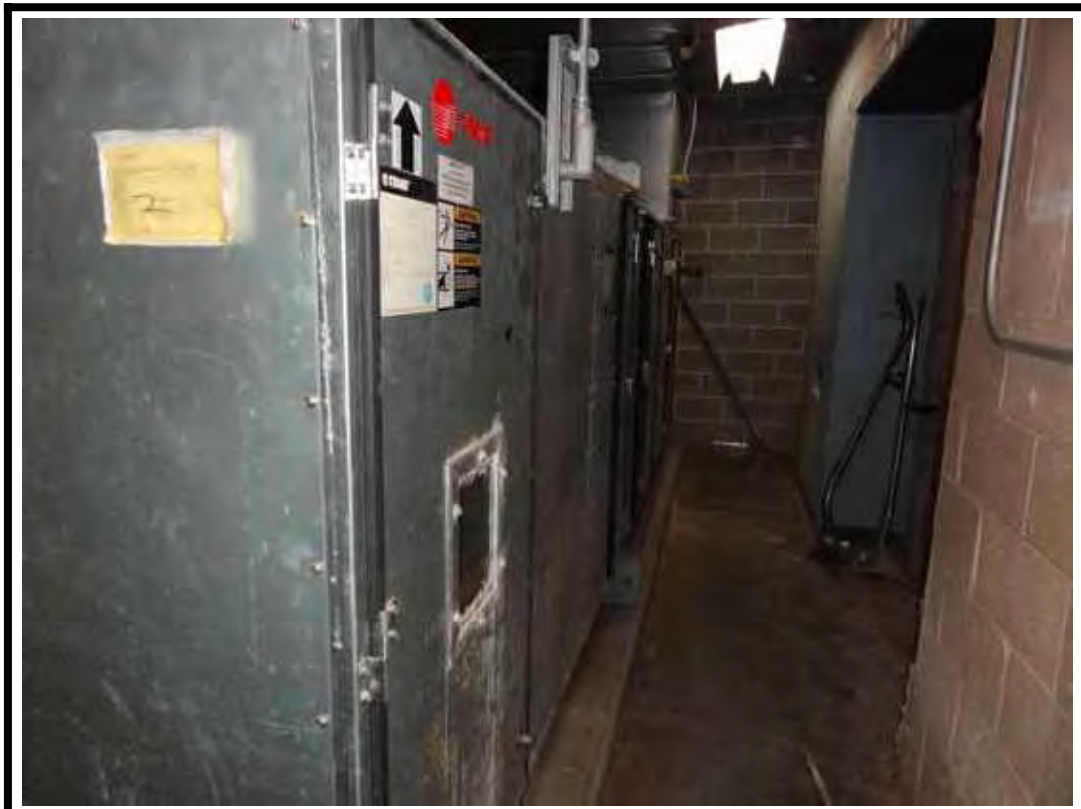
PHOTO NUMBER 4 View of air handling equipment in the janitorial/maintenance closet.
