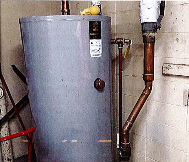
Hot water holding tank
