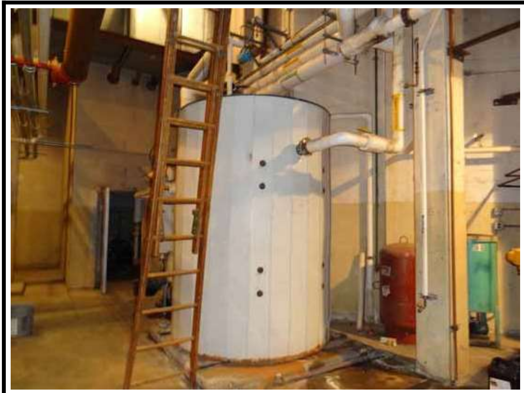
PHOTO NUMBER 65 View of hot water tanks in the subbasement.
