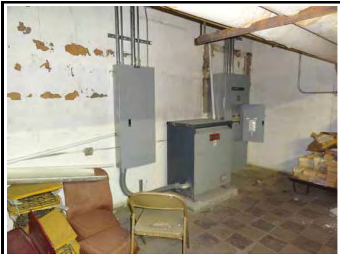
PHOTO NUMBER 50 View of "dry type" transformer in the subbasement.
