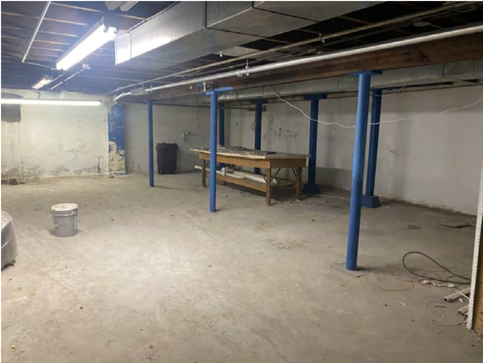
Existing basement area that will provide space for the Community Center Meeting Room
